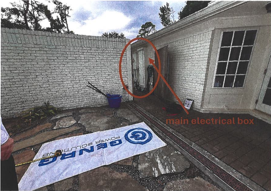
Views of electrical boxes near brick enclosure
