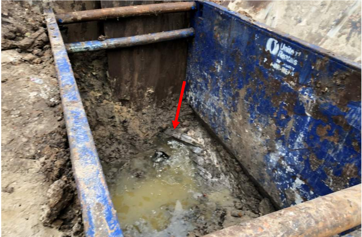
24-inch & 96-inch CMP Damage 12-5-2022
