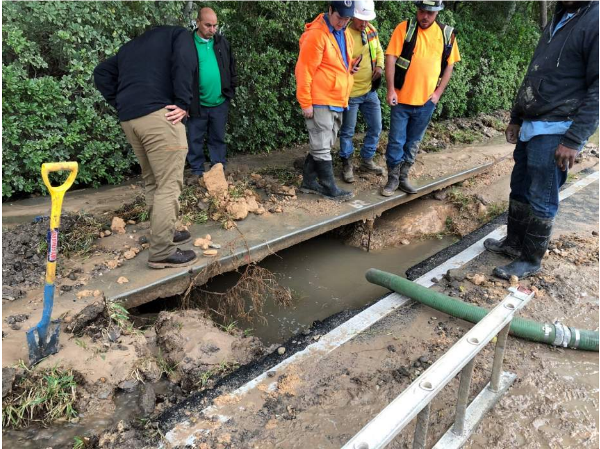
Verizon Water Line Bust Washout 12-1-2022
