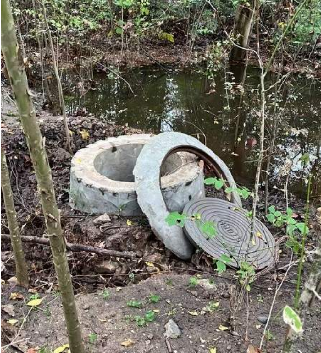
Manhole Cover and Grouted on Ring Blown Off After Rain Event 12-11-2022
