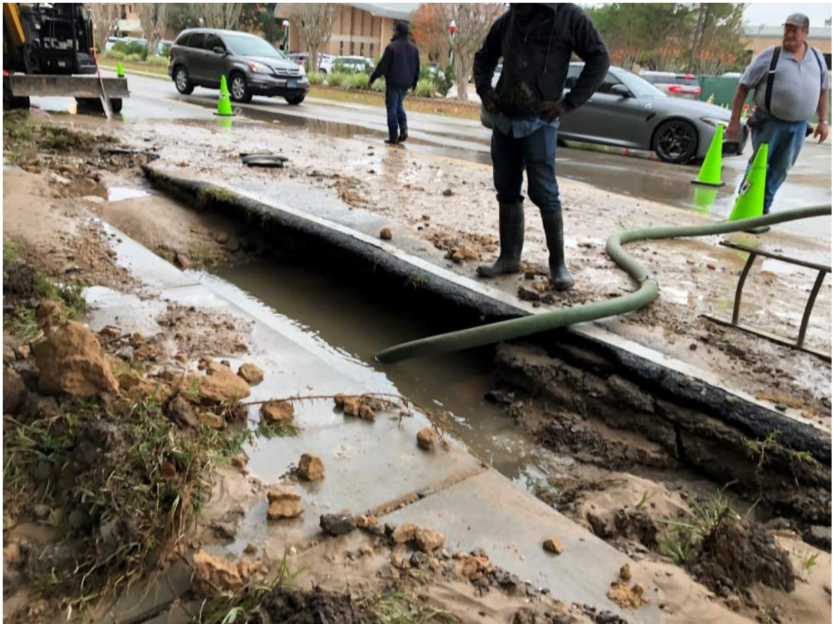
Verizon Water Line Bust Washout 12-1-2022
