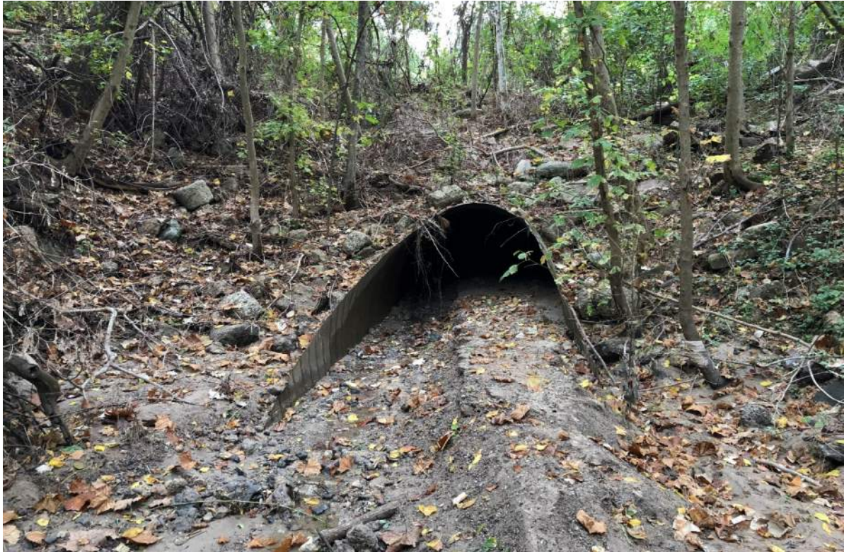
96-inch CMP Outfall: Approximately 50% Full of Soil 12-5-2022
